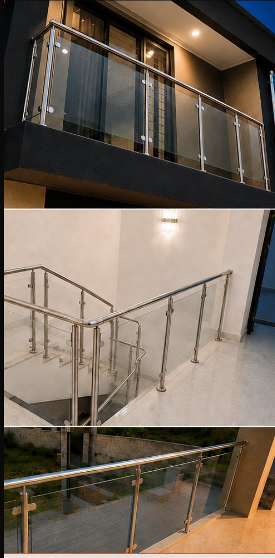
Premium stainless steel and glass balustrade systems installed by Bolide Infrastructure Solutions in Lusaka.
